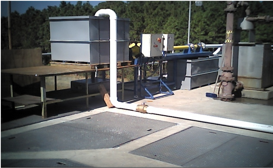
Figure 3 - View of Inlet Pipe and Equalization Tank Feed to VAS Grit Separator
