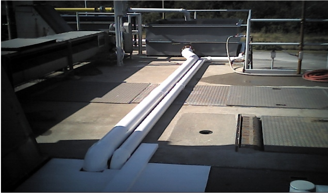
Figure 5 - Discharge Pipes for Return Flow to Northwest Influent Channel
