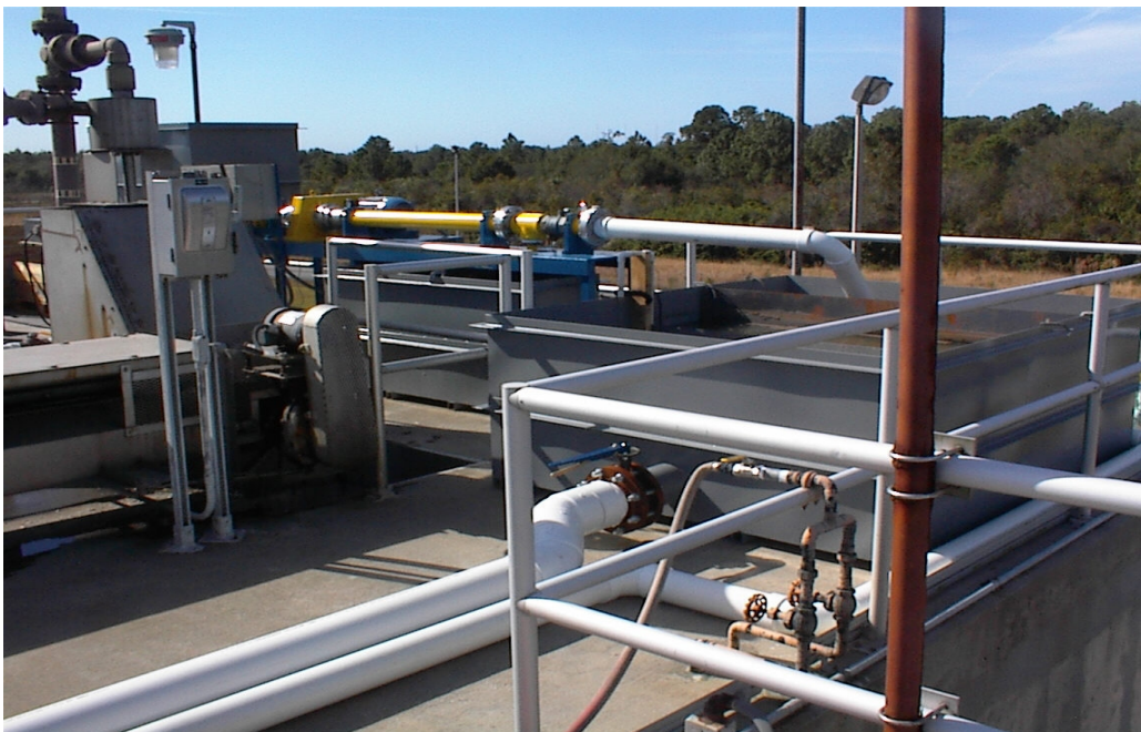
Figure 4 - View of VAS Grit Separator, Grit Collector Tank and Main Tank
